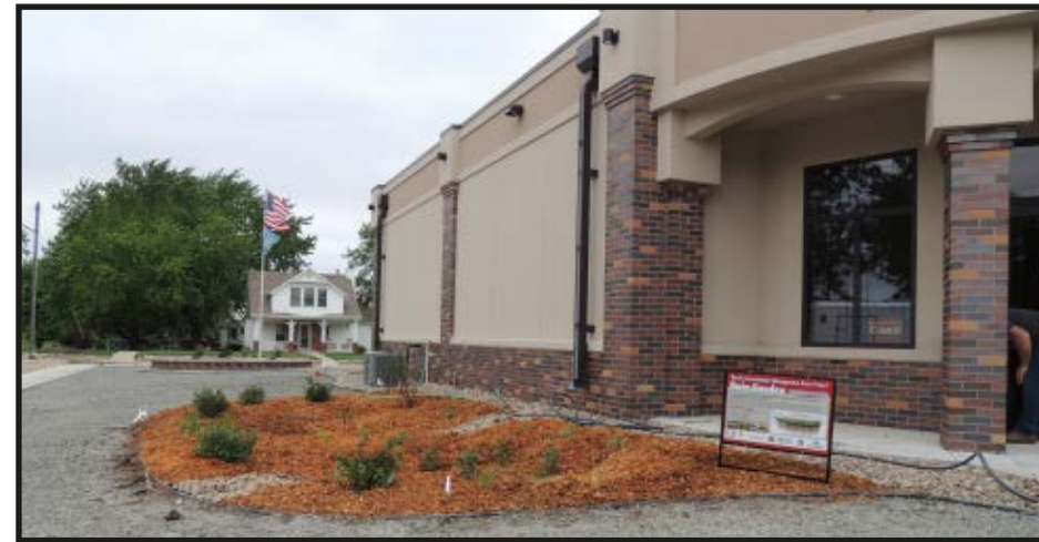
A rain garden was installed in June at the Lied Lincoln Township Library in Wausa, as one of the Bazile Project's urban demonstration sites. Sponsors of the project are: the Lewis & Clark, Lower Elkhorn, Lower Niobrara, and Upper Elkhorn NRDs; and the University of Nebraska Extension. Funding was provided from the Nebraska Environmental Trust and the Nebraska Department of Environmental Quality.
